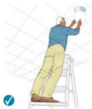
Figure 6b Correct - 3 clear rungs. Don't work any higher up this type of stepladder.
